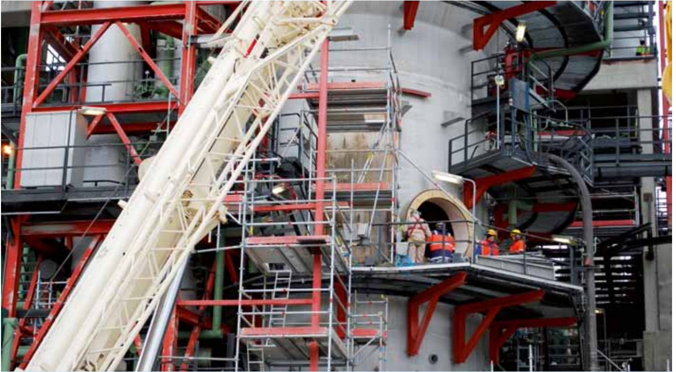
The maintenance turnaround at Porvoo refinery was one of the company's largest investments in 2010.
